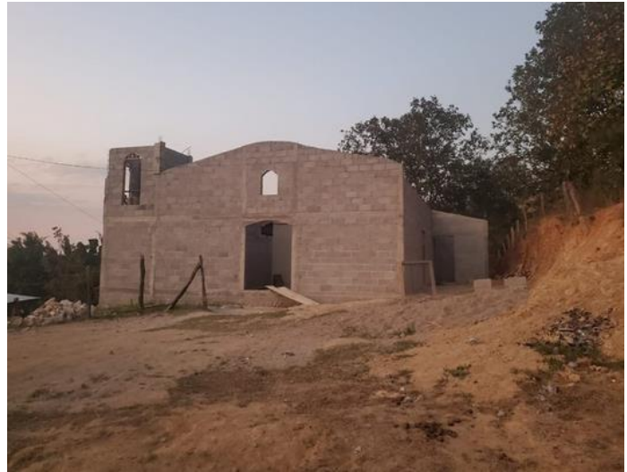
Photograph of the church being built by the leaders of Cedros below Francisco Morazán, Honduras.
